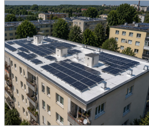
existing buildings with installed PV systems
